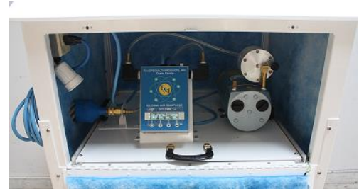
View inside weatherhouse illustrating digital flowmeter
